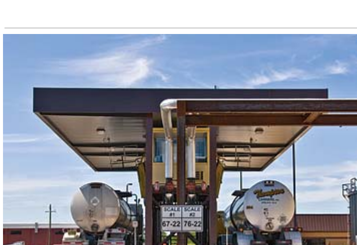
Dual Load-Out Rack The tank truck load-out system is designed so that drivers can safely load the tank truck they are driving without help from others. Two trucks can be filled simultaneously with liquid-asphalt products, each at a rate of 500 gpm. The loading station has a covered roof and an enclosed control room with two sets of operator load-out controls. The system incorporates an overflow device that automatically shuts off the asphalt in case the scales fail to do so when a preset limit is reached.
