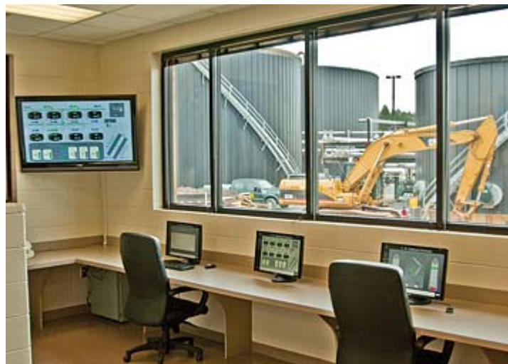
Terminal Office Computers are located at different places in the terminal in order to provide efficient control of all functions. For example: Positions of the three valves on the outlet side of each asphalt pump can be verified on a computer screen before the pump is operated. This view of the terminal office shows the user-friendly design and layout.
