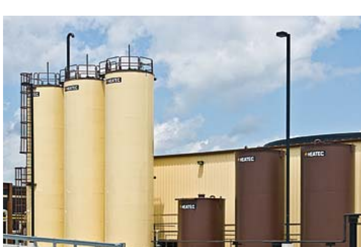
Polymer Let-down Tanks There are three 35,000-gal. tanks that are used to store finished PMA (polymer modified asphalt) at the Rockmart Terminal.
