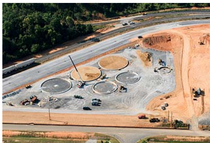
This is an aerial view of the site when the construction work had just been started. The photo was taken on July 2, 2008. Compare it with the aerial photo above. That one was taken on June 26, 2009.
