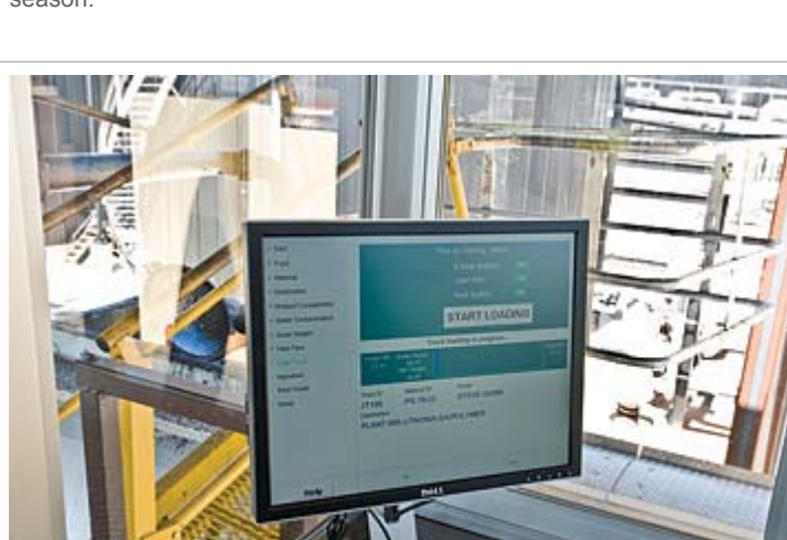
Computer at Load-Out Rack The load-out system incorporates a computer, computer-automated controls, two truck scales, and automated data recording. The automated controls provide remote operation of the asphalt pumps located at the tanks. The load-out controls for each load-out boom incorporates lockouts to prevent operation of the pumps unless the boom is properly positioned and valves are properly set. The components of the truck scales and the load-out system were provided by Astec.
