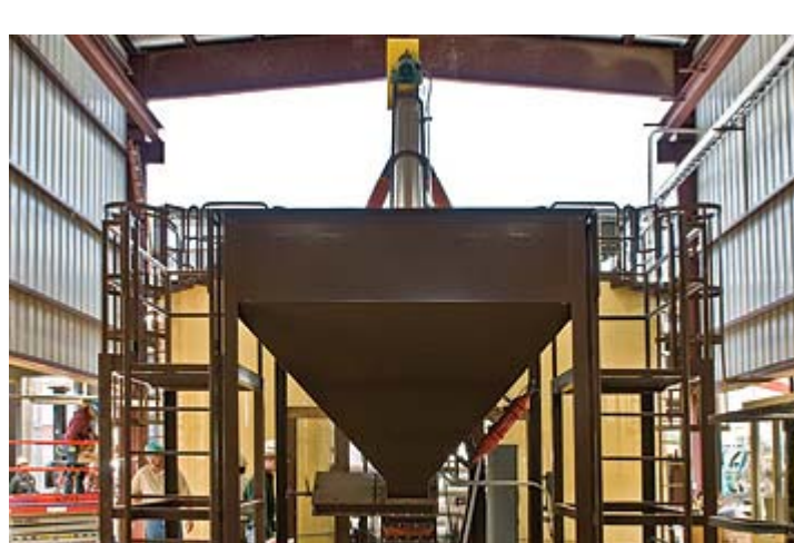
Polymer Blending System The terminal has a separate building that was constructed specifically for housing the equipment needed in the company's polymer blending operations. In the foreground of this photo is the hopper where polymer pellets are loaded. The two tanks in the background are used to mix the polymer with liquid AC. According to a Heatec spokesman, C.W. Matthews Contracting will have processed more than 20,000 tons of polymer mix in the months between May 2009 and the end of the paving season.
